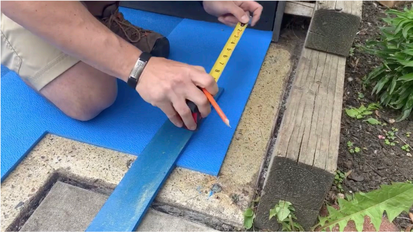
Step 27: Measure and mark to continue the staggered pattern with Transition Strips.
