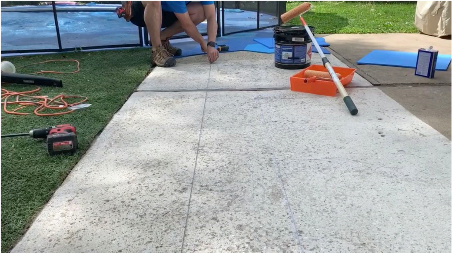
Step 7: Measure and snap lines 12" off the center line on both sides. The 12" offset line will determine the starting point for the installation.
