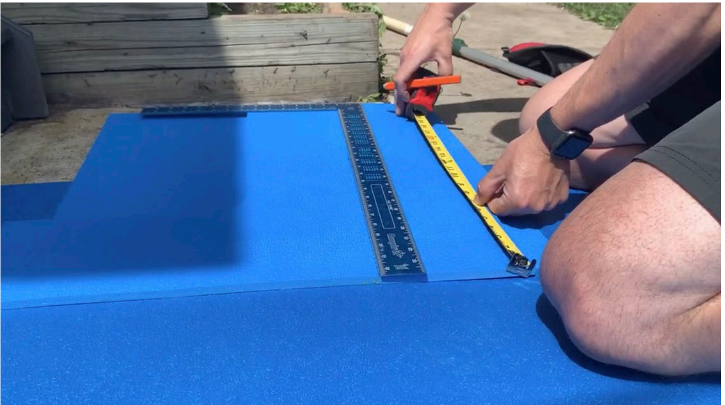
Step 8: Measure the length of the infill piece and mark the tile. Connect the points using a straight edge to create cut lines.
