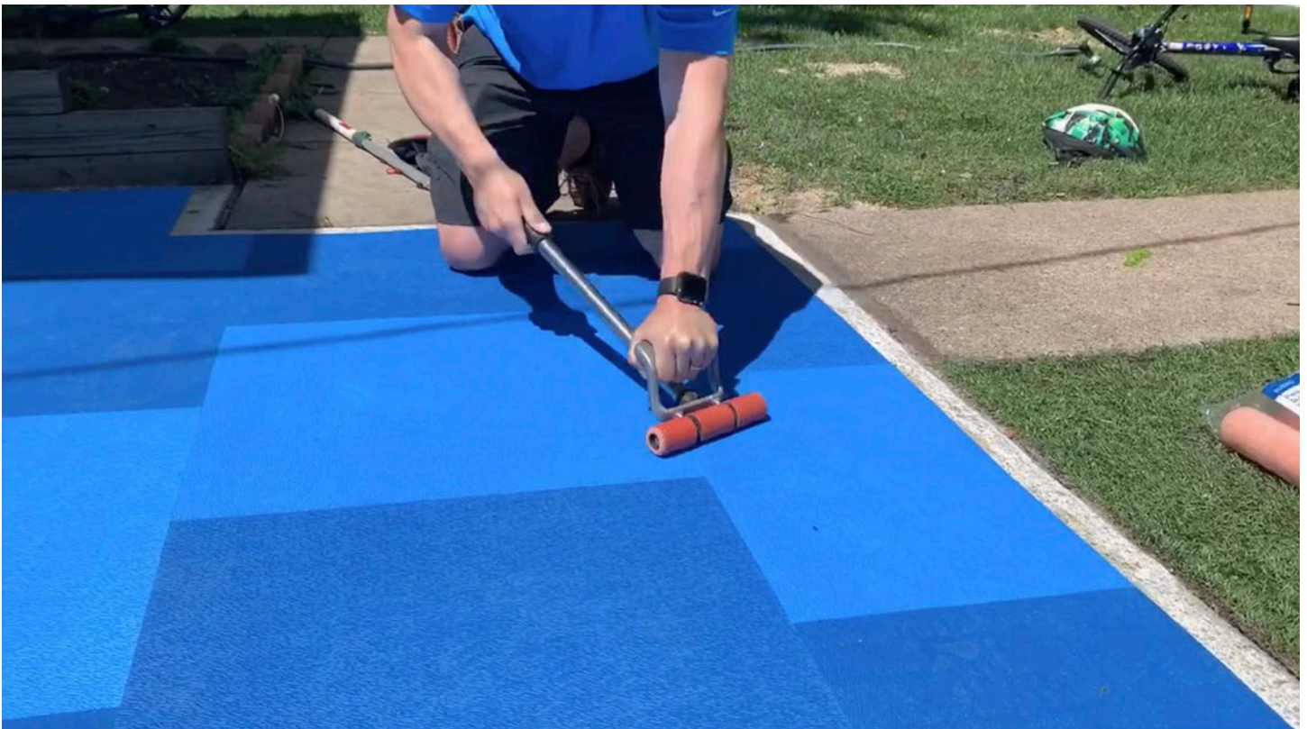
Step 24: Once the excess tile has been removed from the edges, use a hand roller to work down all remaining tiles. The smaller size helps to press the tile into the adhesive bond.
