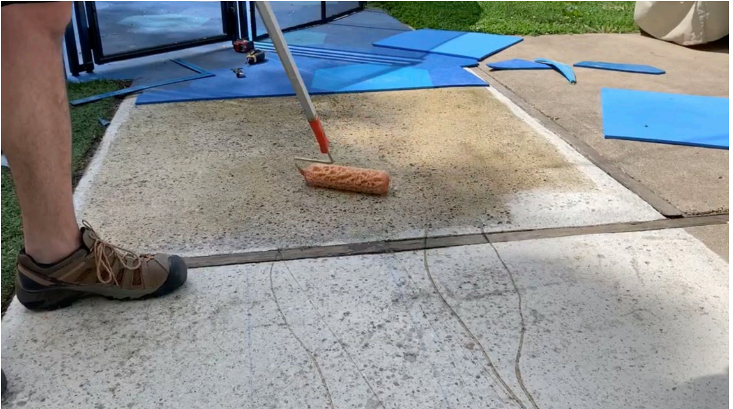
For the main portion of the install area, apply adhesive with a pole extension on the roller frame. Cover the concrete thoroughly with complete and even adhesive coverage.
