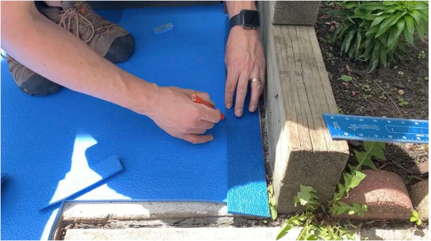
Step 18: Lay out Transition Strips by placing them along the perimeter of the concrete and marking where they land on the tiles. These edges will need to be trimmed.
