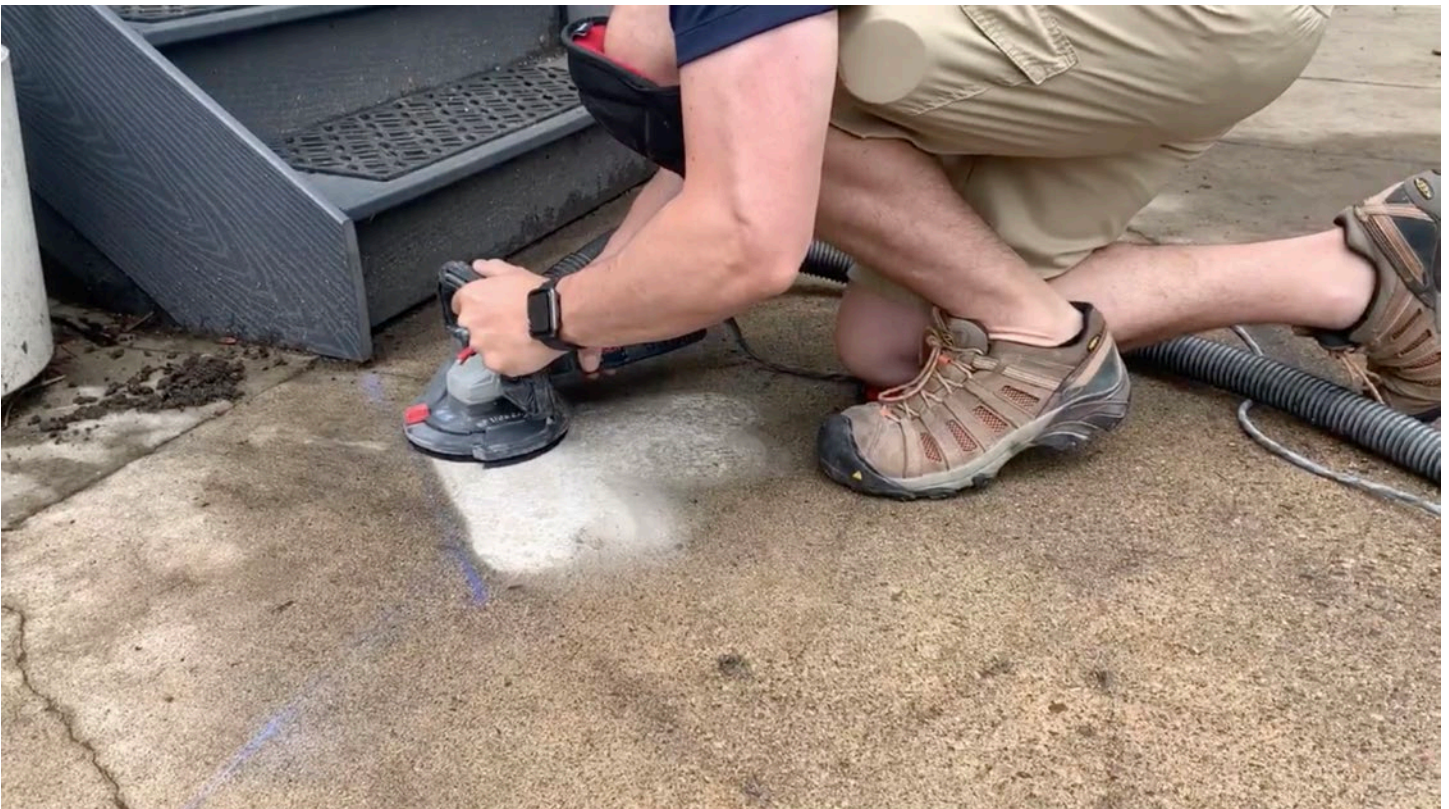
Step 2: Grind the concrete. Grind just up to the chalk line to prepare the area that will receive Life Floor. Grinding down the top layer of the concrete allows for proper adhesion.
