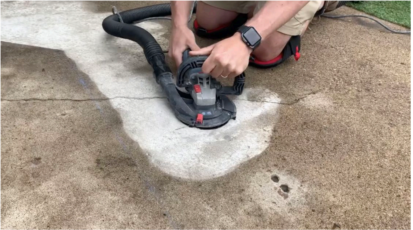
Completely grind through the top layer of the concrete to reveal the clean slab below.
