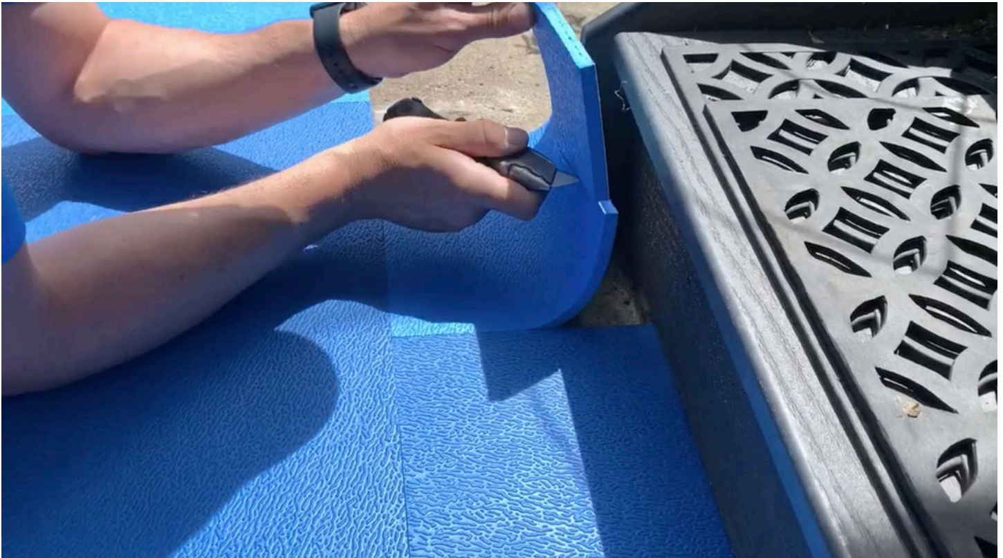
Step 14: Using a similar method, place the tile piece, ensure a tight joint at the edge, and roughly cut off the excess while leaving the tile a little long.
