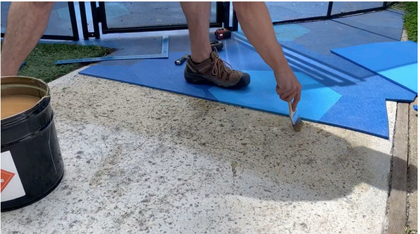
Step 4: Use a 3" chip brush to distribute adhesive along the edges, being careful to only coat the concrete slab. Prevent the adhesive from touching any existing materials or tiles.
