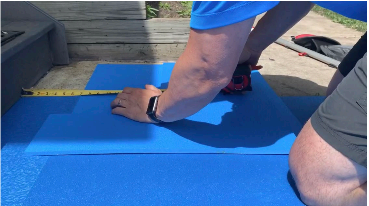
Step 6: As a different method to fill in the gap, measure the depth of the concrete at both sides.
