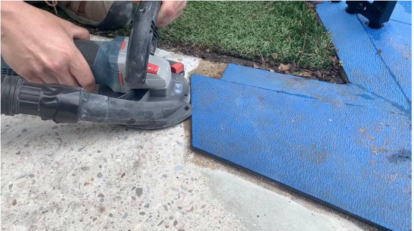
Grind right up to the edge of any pre-existing tiles. Move back the guard of the grinder to remove the top layer of the concrete at the tile edge.
