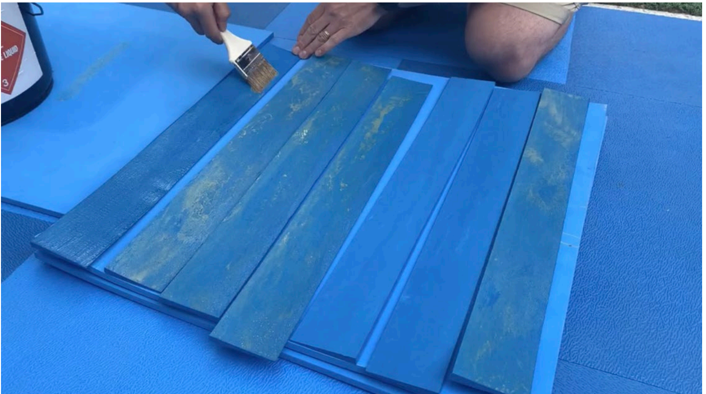
Step 26: Apply the adhesive to bottoms of Transition Strips using a brush. Ensure even and complete coverage on each portion, ensuring adhesive does not get on the sides of the strips.
