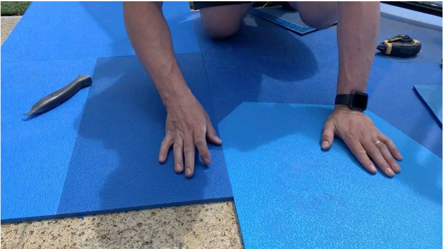
Step 11: Work the edge of the tile into the joint and down onto the concrete to ensure a tight fit.
