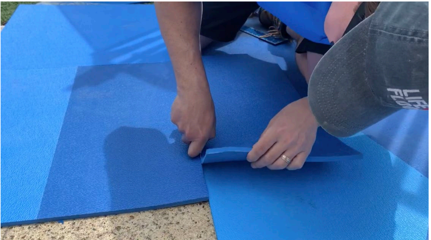
Step 10: Cut through the top tile and run the blade along the existing edge. Be careful to only cut into the top tile while pulling away the excess with your opposite hand.
