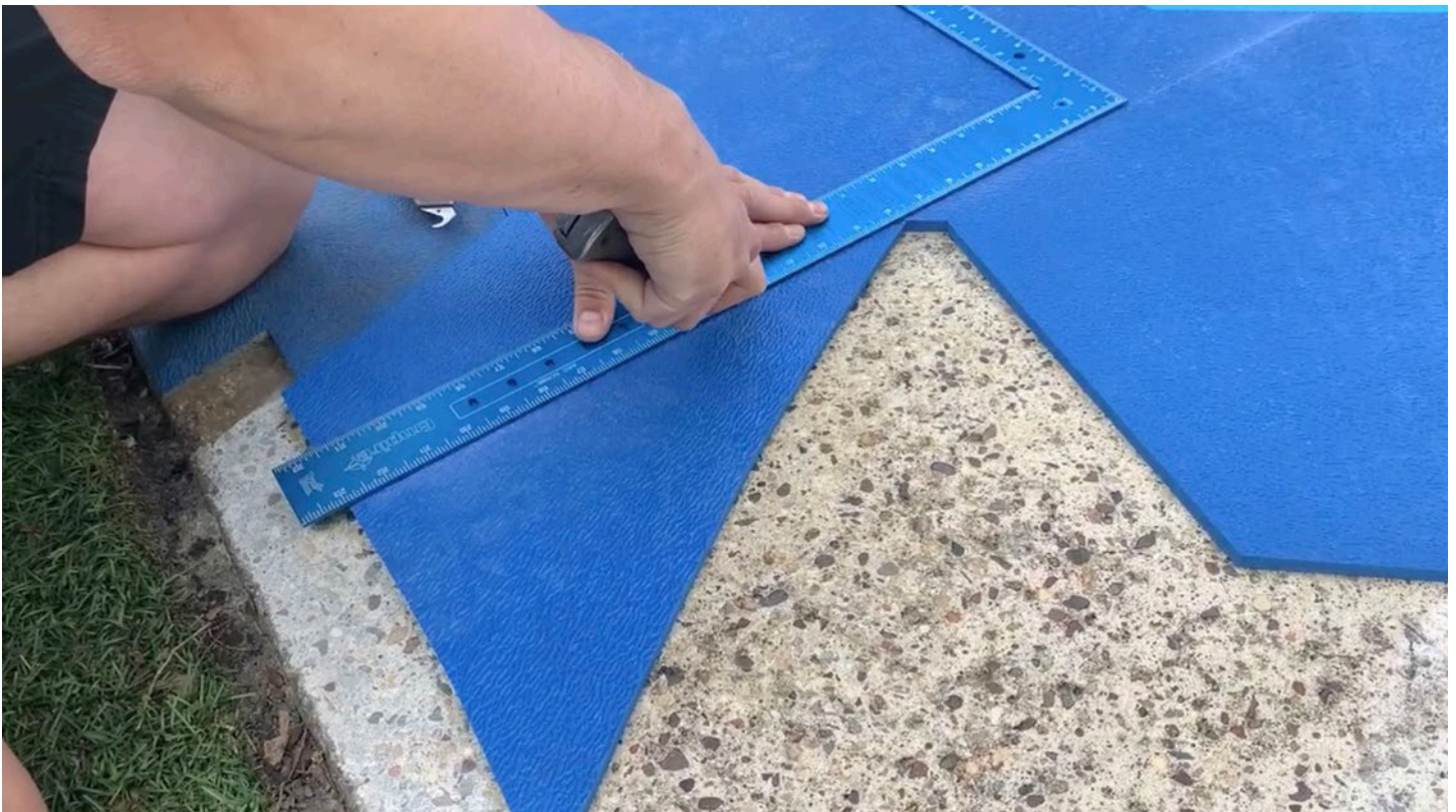
For the project shown here, a line was snapped to create a cut line along existing hexagon tiles and prepare a clean tie-in point for the new square tiles.
