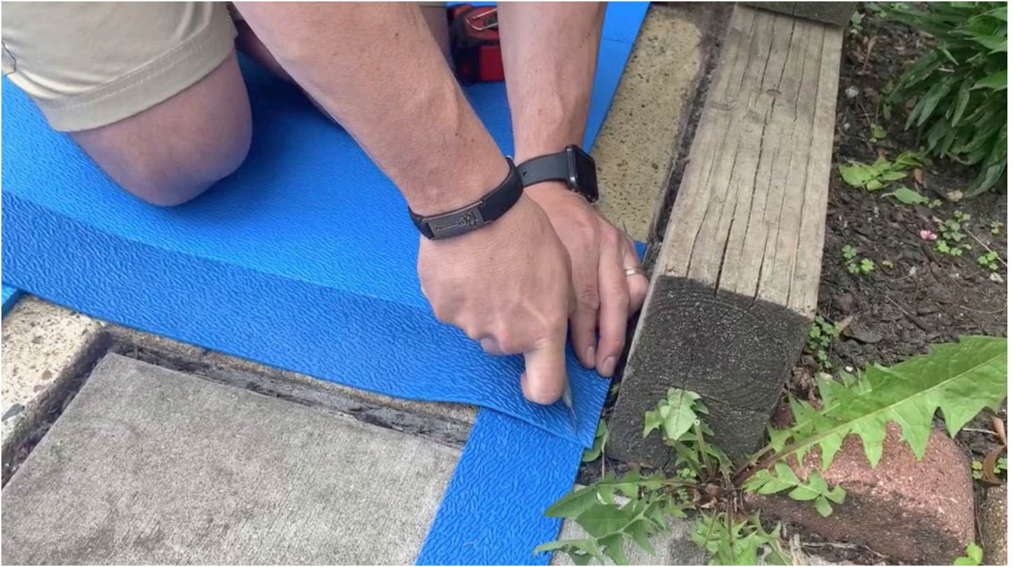
Step 31: Overlap both Transition Strips and cut through them at the corner simultaneously to create the miter. You can also measure using a speed square.
