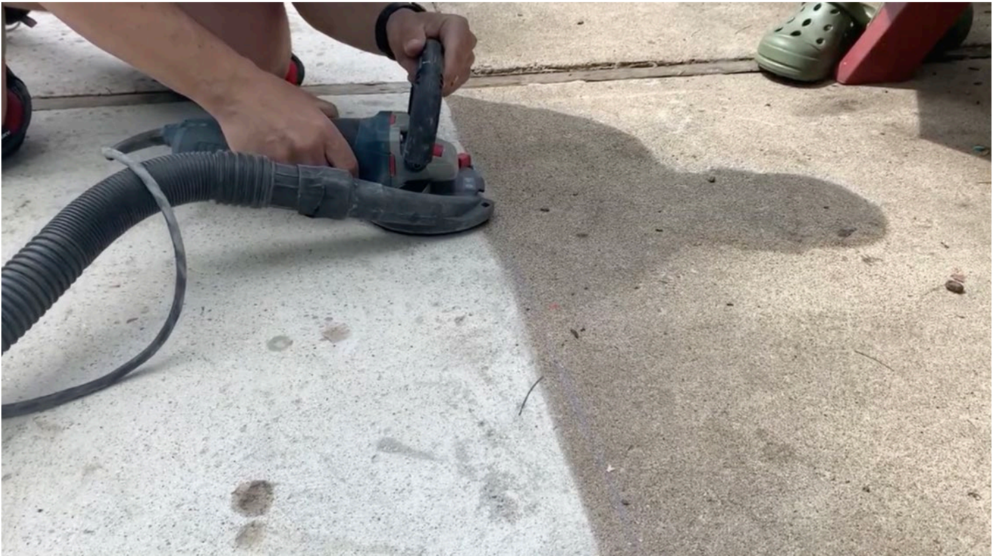
Grinding is complete once the whole surface that will receive tiles has been addressed, making sure to grind up to all edges and chalk lines of the project area.
