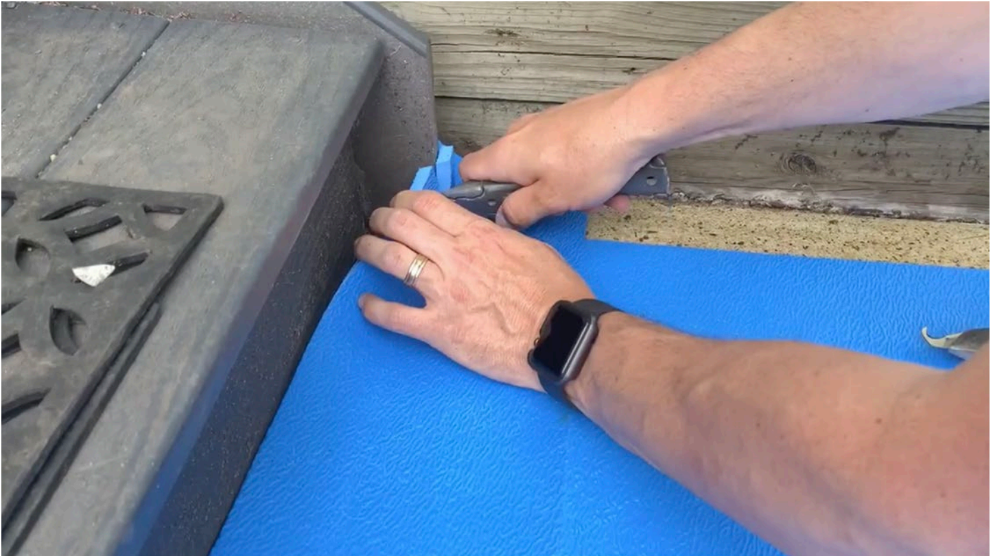
Step 11: Run straight blade along edges of bump-out to cut tile on either side.
