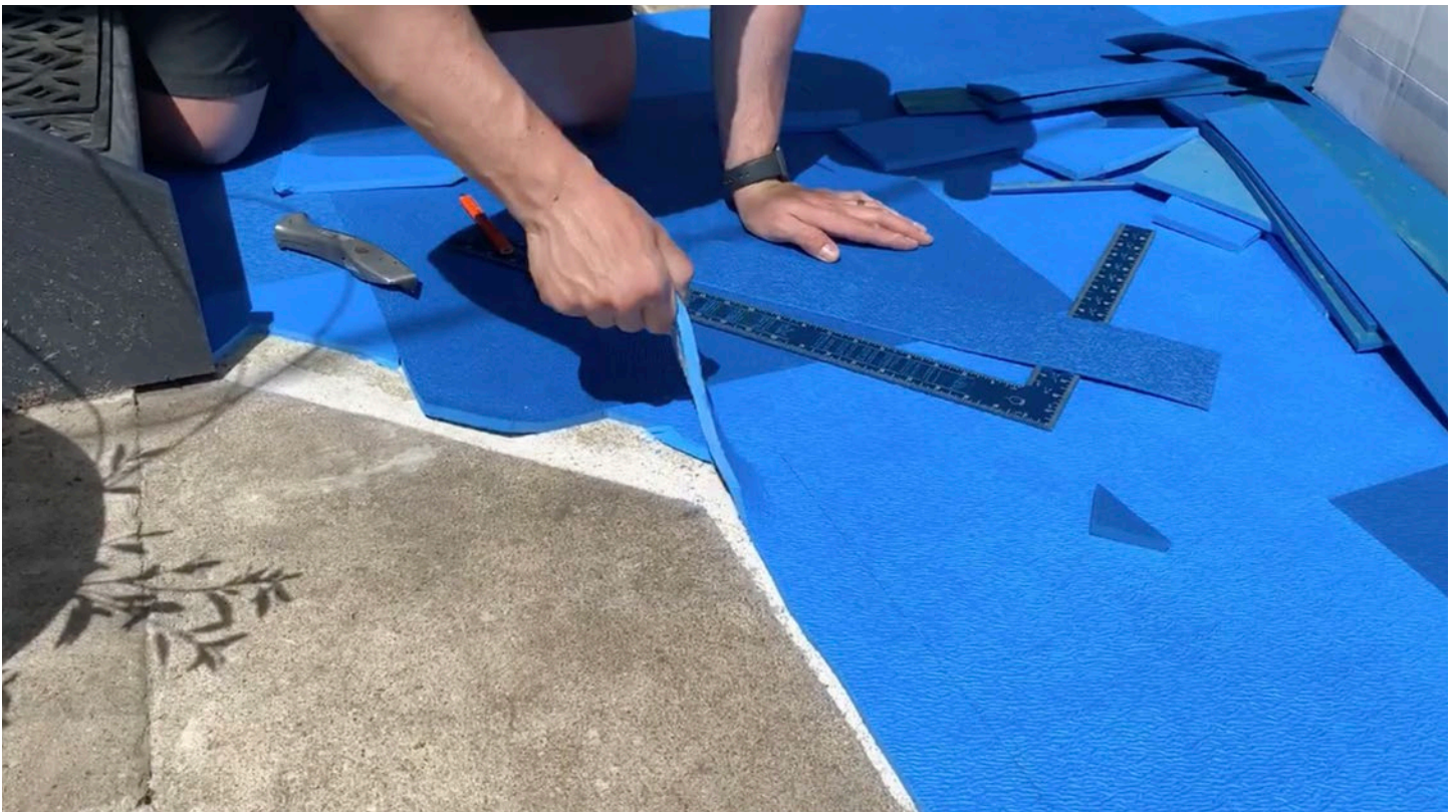
Step 22: Pull away excess tile to prep for Transition Strips. Limiting adhesive at the edges earlier in the process prevents the need for intensive tear-out.
