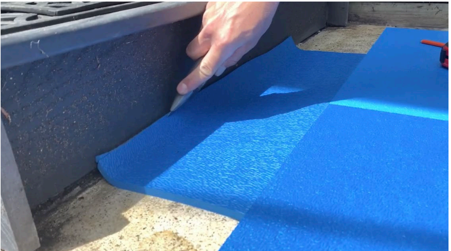
Step 4: There's a gap below this stair riser, so this piece is freehand cut a little long. A hook blade is used to ensure that only the Life Floor tile is cut in the process.
