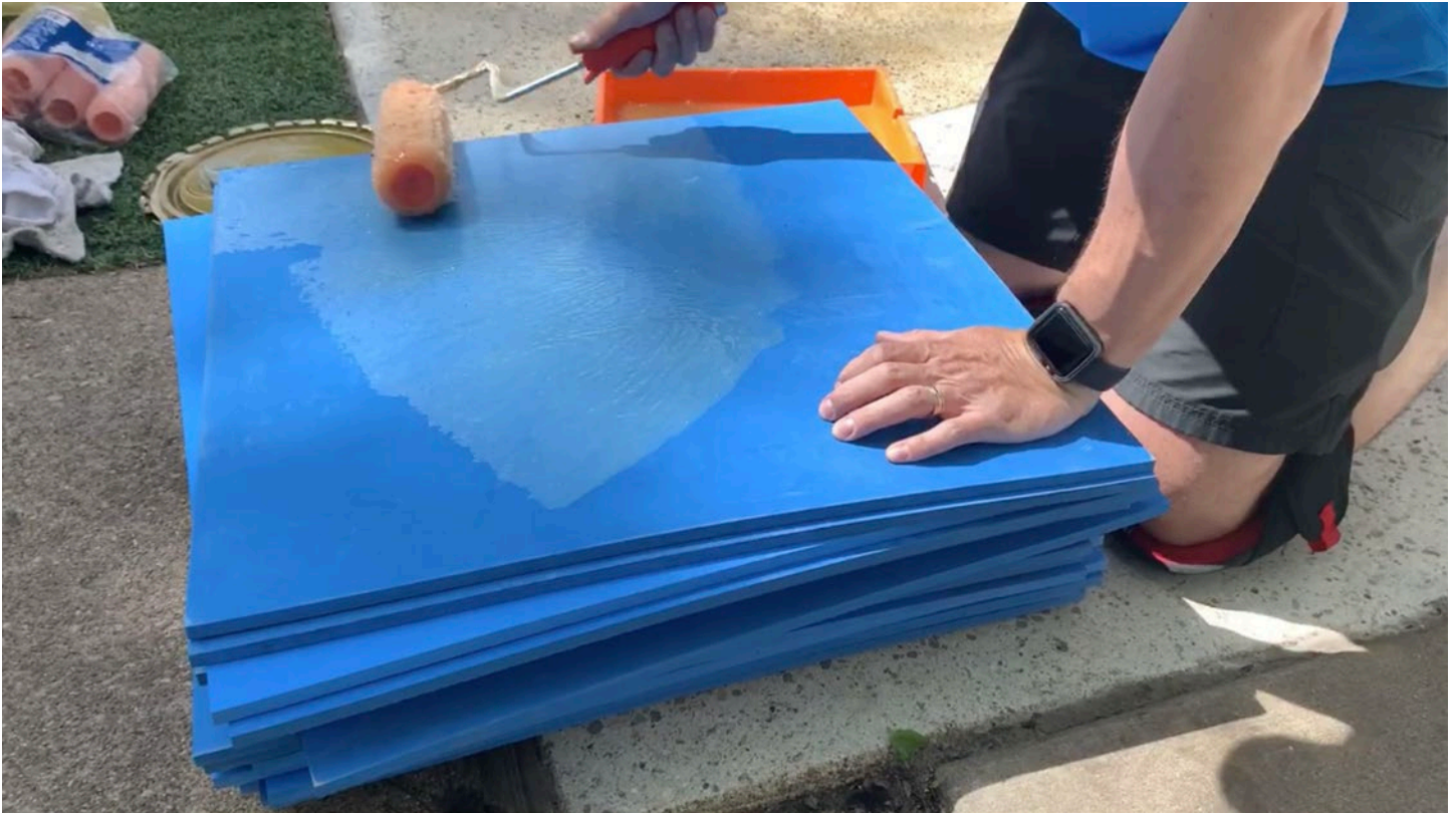
Step 5: Work out of the tray to apply adhesive to the backs of the tiles. Start from the middle and work to the edges for 100% coverage. Avoid the sides and top faces of the tiles.
