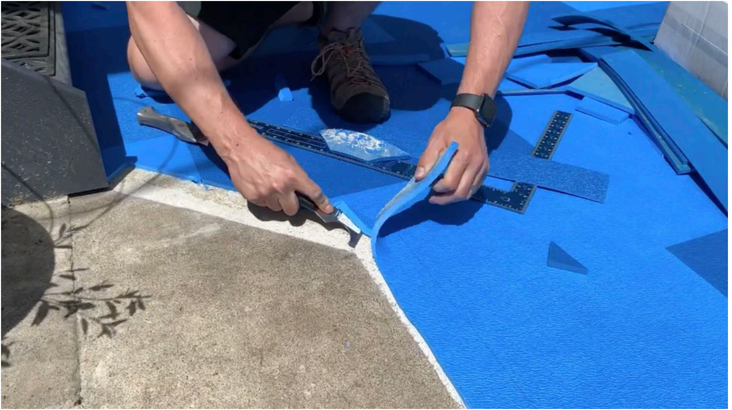
Step 23: Use a 5-in-1 tool to remove excess tile that is glued down. Continue this process around the entire project perimeter.
