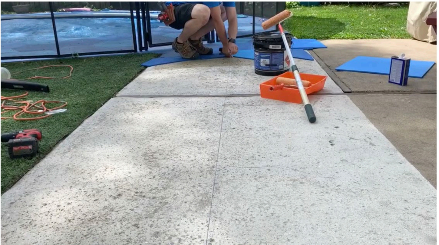
Step 6: Measure and mark the center points of the slab at opposite edges and connect the points by snapping a center line across the project area.
