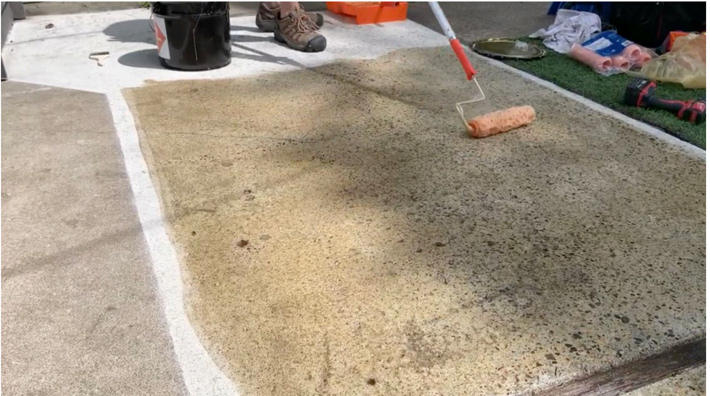
The roller can be dipped directly in the adhesive can, but avoid debris like leaves getting into it. Ensure complete coverage and leave a 3" margin at the edges where Transition Strips will be applied later.
